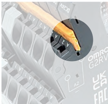
Electrical shock hazard
